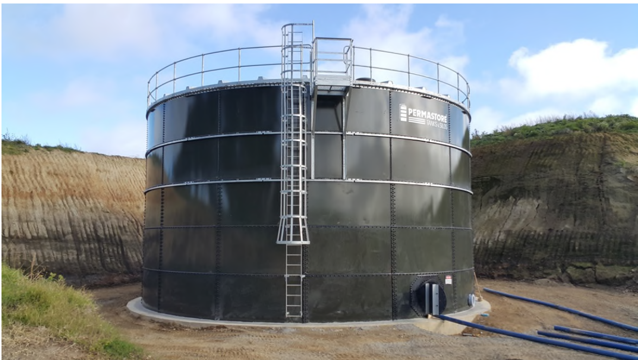
New Rātana water reservoir
