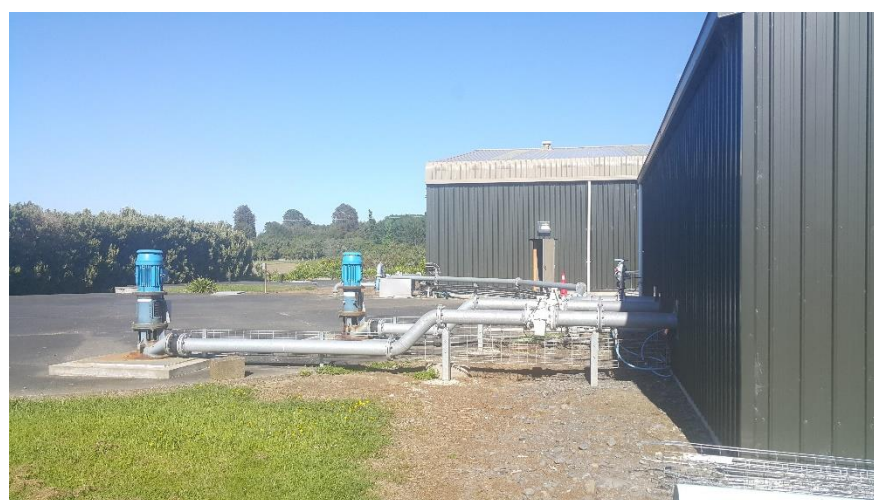
Images: Marton Wastewater Treatment Plant
