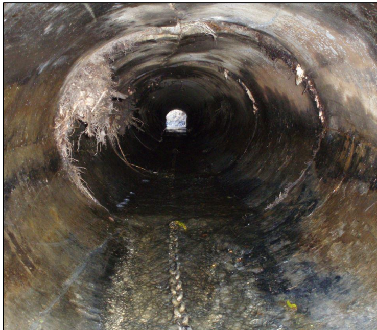
Figure 43: Large Culvert Approaching End of Useful Life
