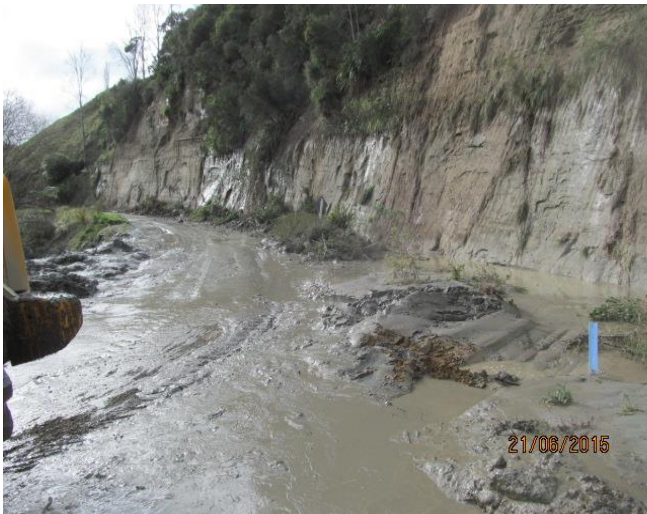
Turakina Valley Road under flood waters
