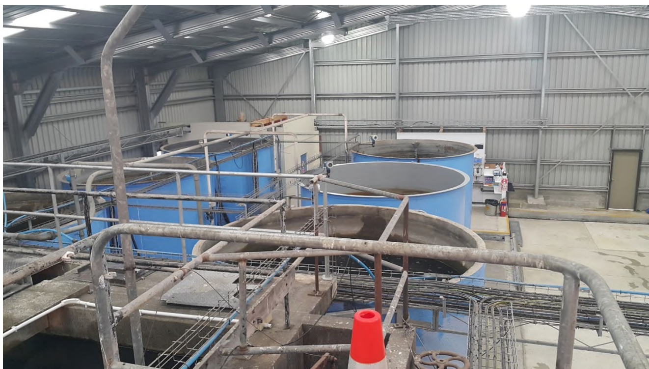
Water treatment tanks, Marton
