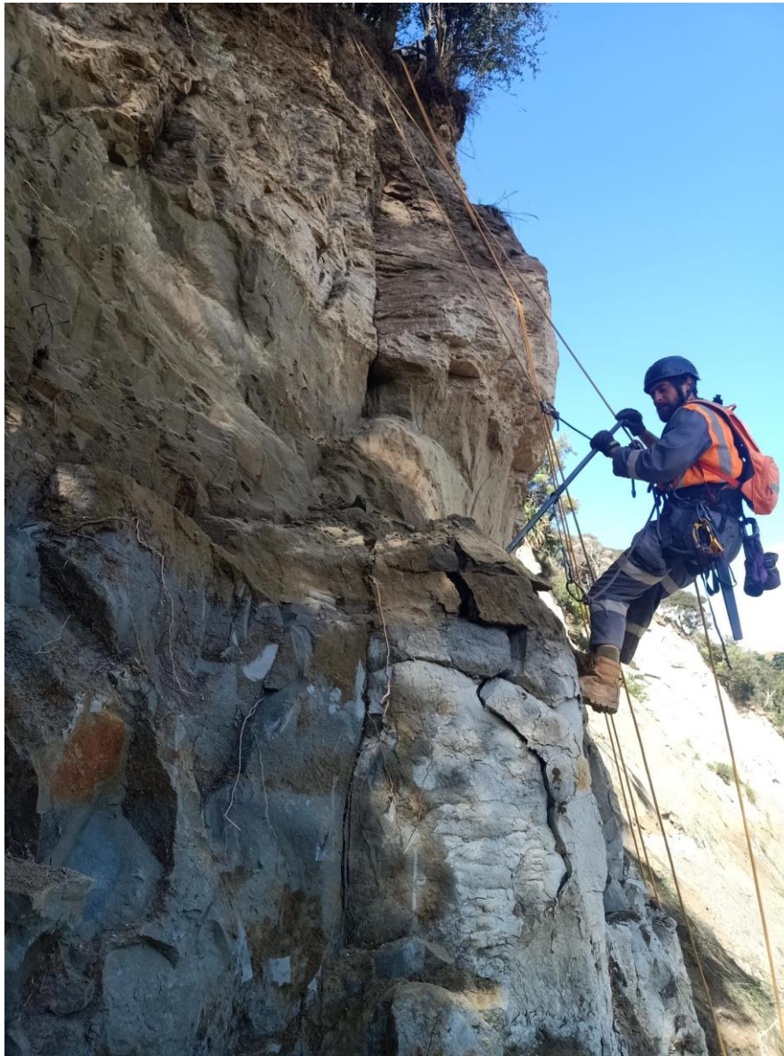
Photo: removing loose material from the face of the Okirae Bluff using a crowbar – 24 March 22.
