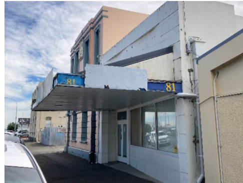
Deteriorating building. Childers Rd
