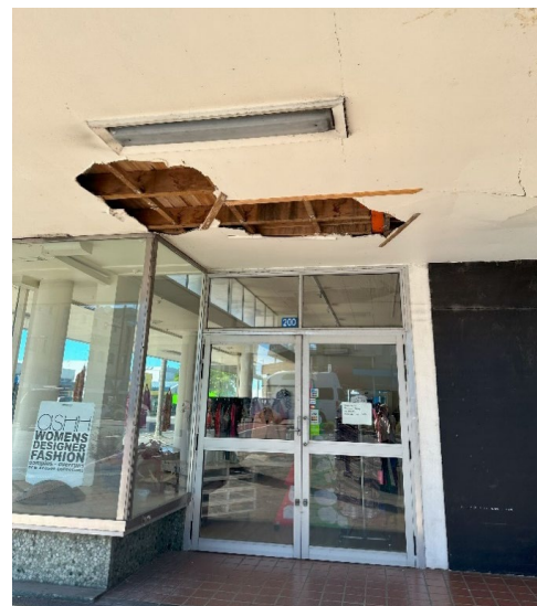
Main Street building decay. Gladstone Rd
