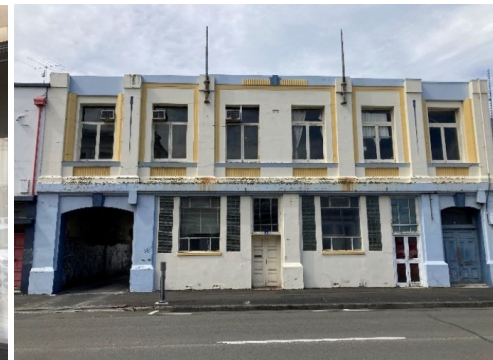
Deteriorating building. Lowe St
