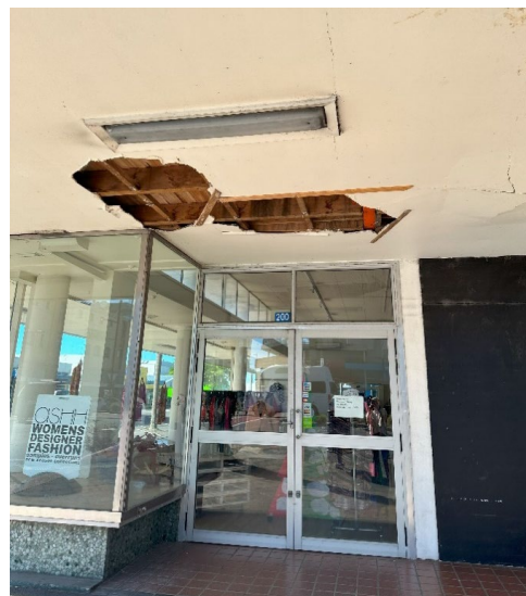
Main Street building decay. Gladstone Rd
