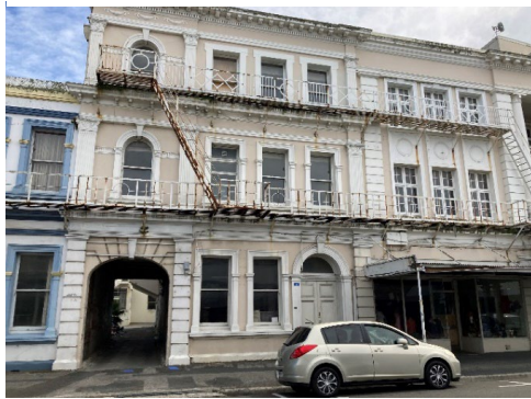
Masonic Hotel decaying façade. Lowe St
