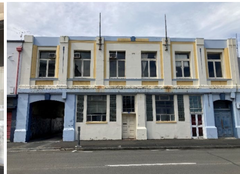
Deteriorating building. Lowe St
