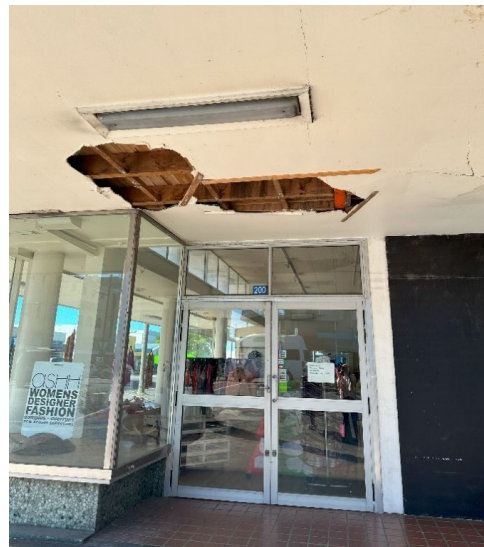
Main Street building decay. Gladstone Rd
