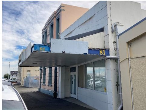
Deteriorating building. Childers Rd
