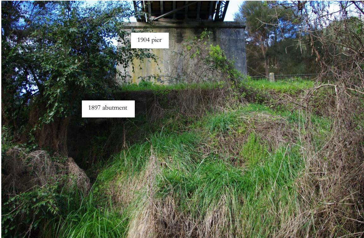
Figure 34: 1897 abutment on eastern side of the river viewed from below, with 1904 pier in background
