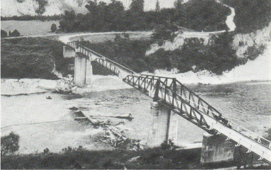
Figure 21: Wash out of low level bridge (reproduced from Laurenson 1979)
