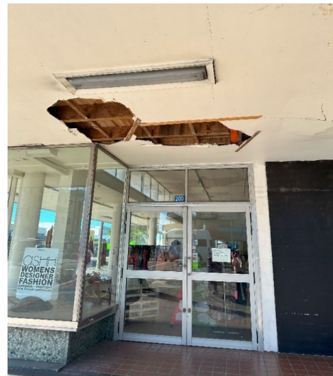
Main Street building decay. Gladstone Rd
