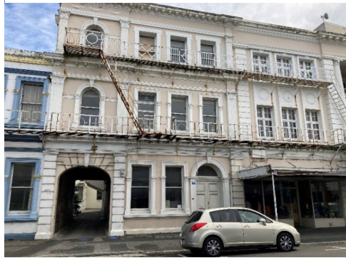
Masonic Hotel decaying façade. Lowe St
