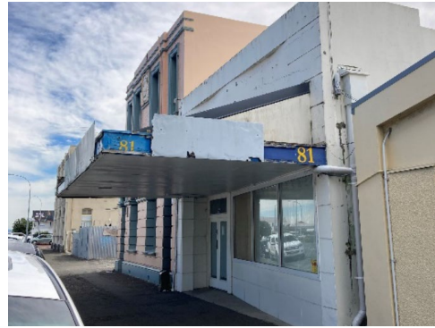
Deteriorating building. Childers Rd
