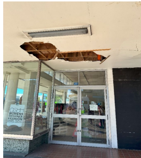
Main Street building decay. Gladstone Rd
